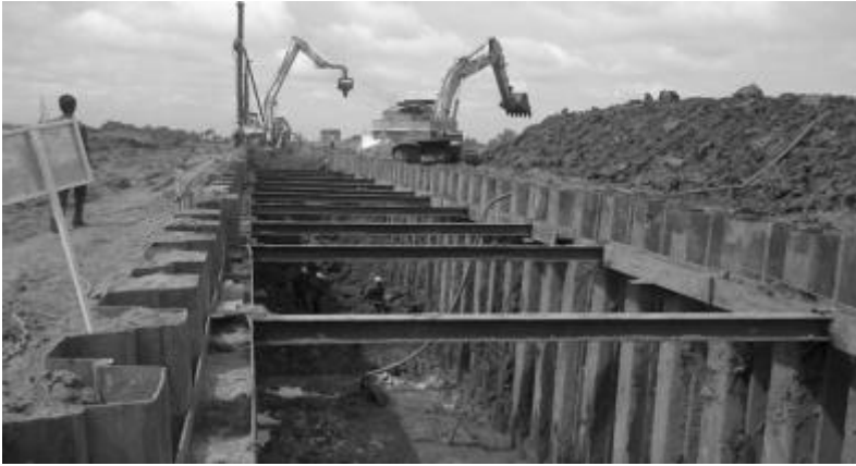
Figure 14. Trench protection: With heavy construction plants operating next to the trench, the excavation had to be protected from collapse. Once the underground pipe was laid the sheet piles are then removed and used on another construction site.
