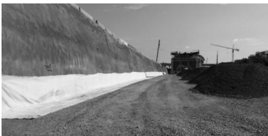
Figure 4. A typical cross section of MSE Walls 6 and 7 as well as the temporary soil nail wall
