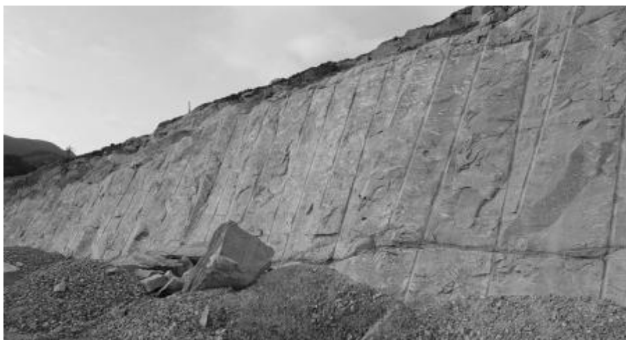
Figure 2. Very hard rock with little jointing at the box-cut where soil nail spacing was increased
